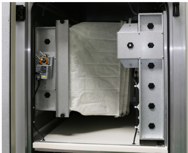
Filter in de unit.
