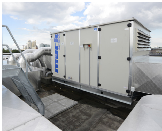
AIRSTREAM wtw-units in buitenopstelling.
