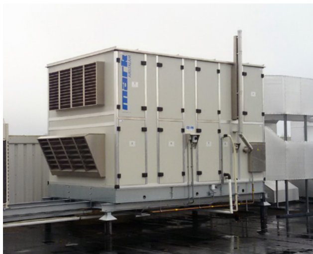
AIRSTREAM wtw-unit in buitenopstelling.
