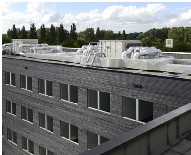
AIRSTREAM wtw-units in buitenopstelling.
