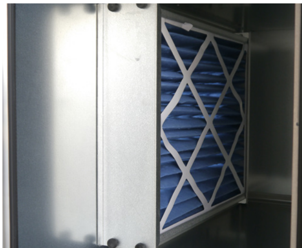
Filter in de unit.
