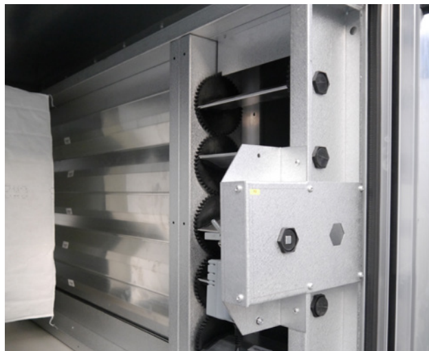
Bypass in de unit.
